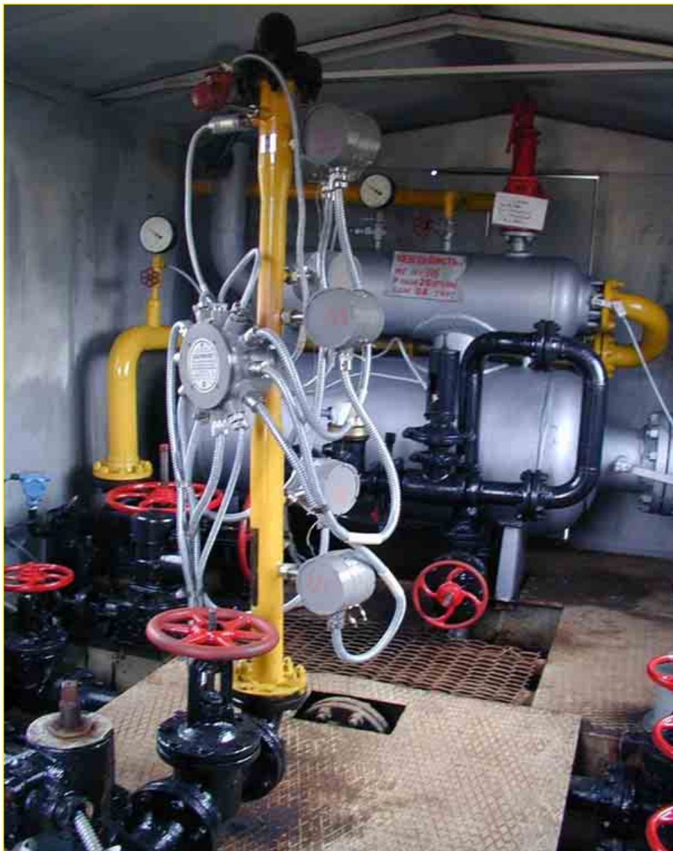
Fig. 10. Multiphase flow meter "Ultraflow" connected in series with measuring system "Sputnik".
